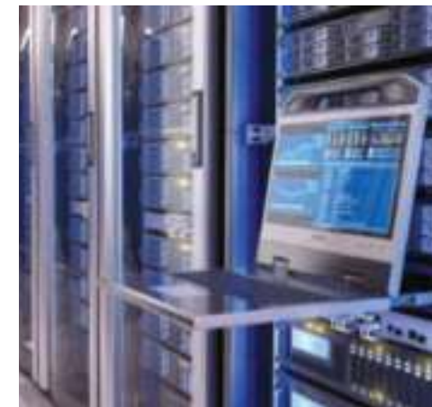
Server Room / Server Rack
