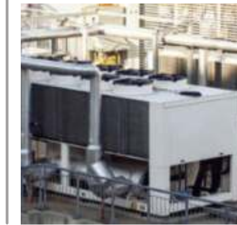
Chilled Water System
