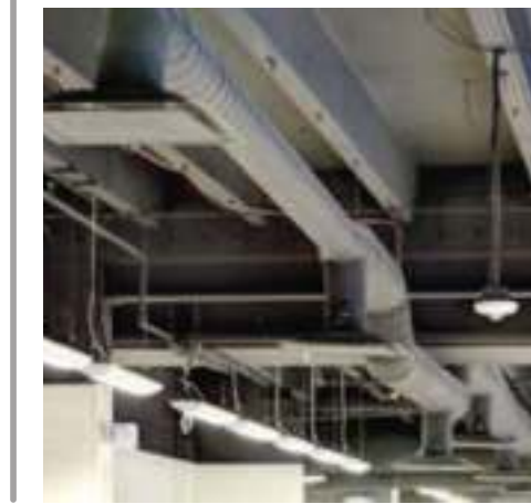
AC and Fire rated Ducts Works
